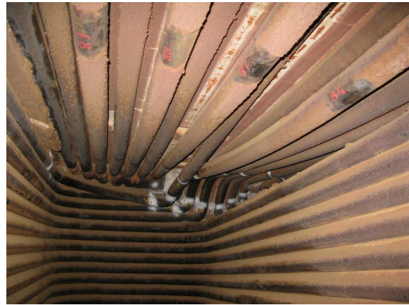
Distortion of tubes in a thermal oil heater, caused in part because there were no backup batteries for portion of the distributed control system.
