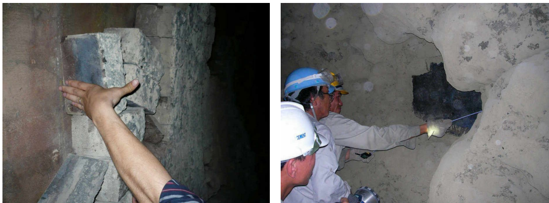
An engineer at a cement factory in Vietnam, that had had a series of stoppages because of power failures. Left: illustrating how much a brick has been reduced in thickness. Right: looking at a hole in the refractory that would otherwise protect the steel shell. The localized loss of refractory caused the kiln to glow red on the outside.
